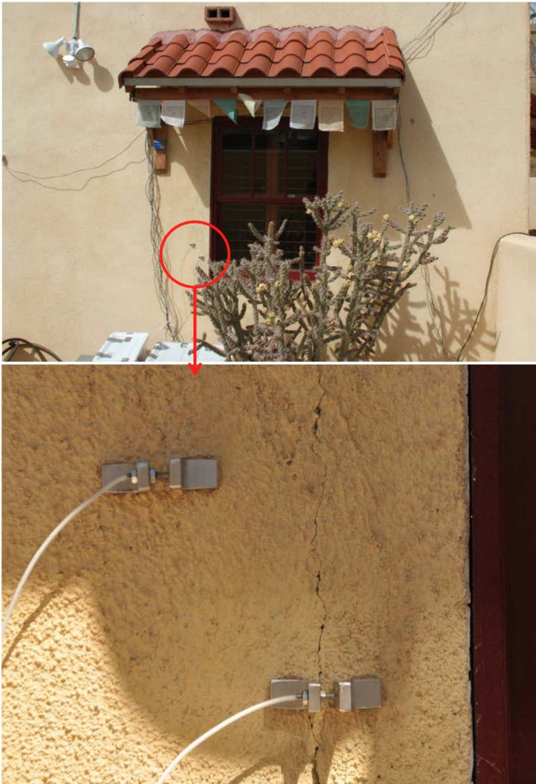
Figure AB-4 - Crack displacement gauges mounted over an existing crack and un-cracked wall section
